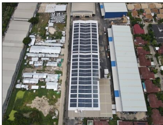
Picture 1: Solar Rooftop Project, Phase 2, Samut Prakan Factory.
